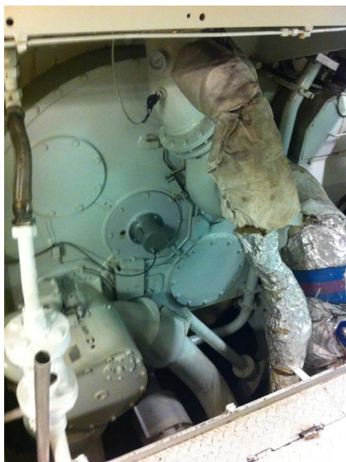
CPS mounted on engine / in engine room
